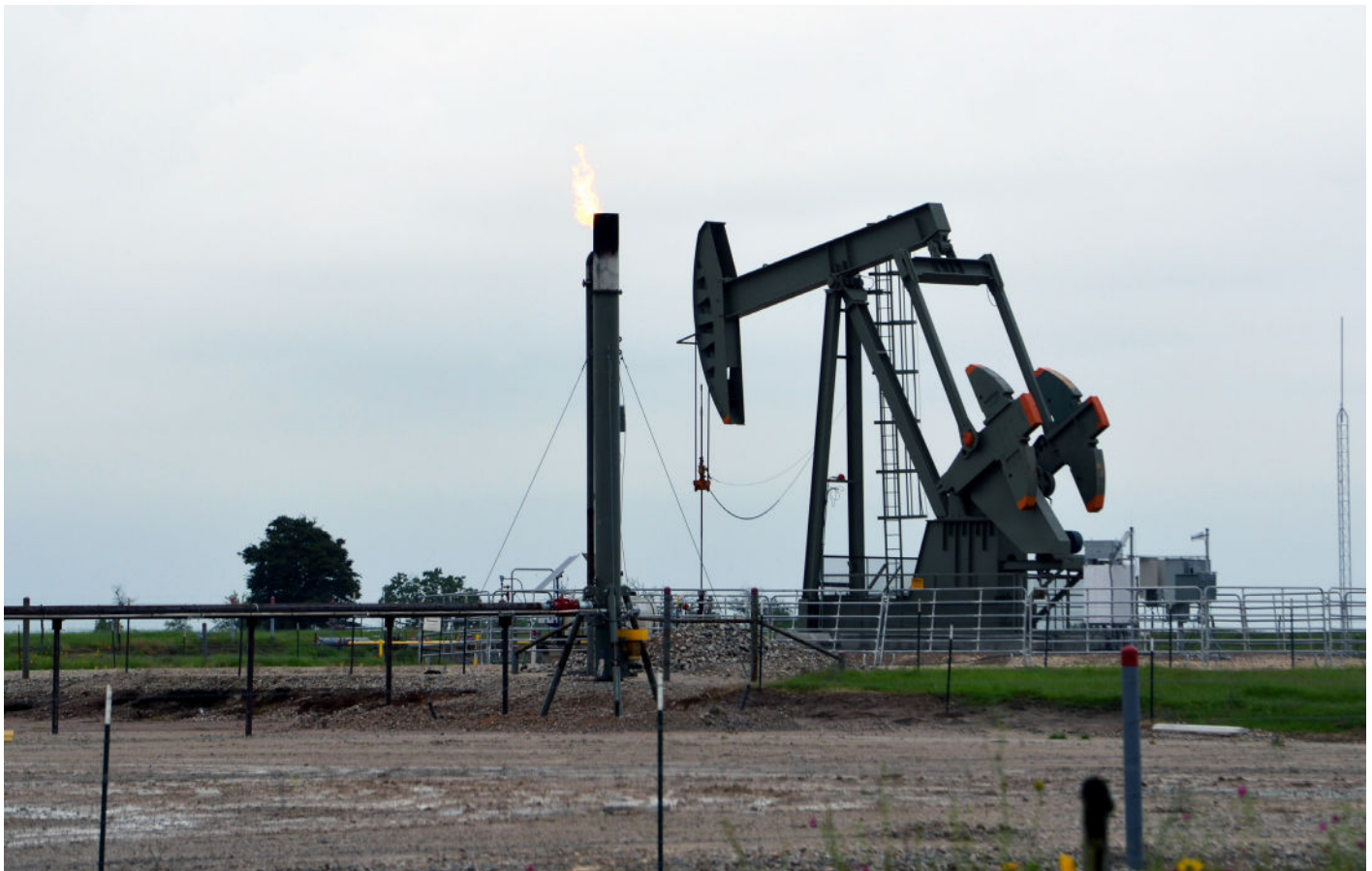
Pump jack and flare in Eagle Ford Shale in South Texas, May 2015. Photo credit: Earthworks
